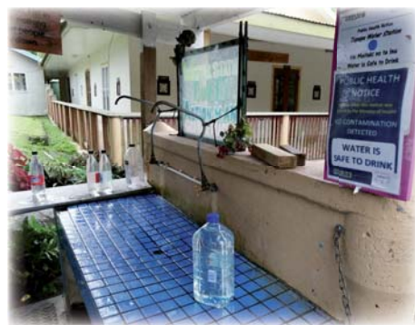
One of the local water filter stations
